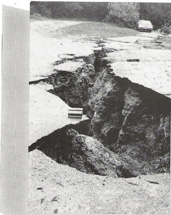
One "BIG" crack on Summit Drive.
