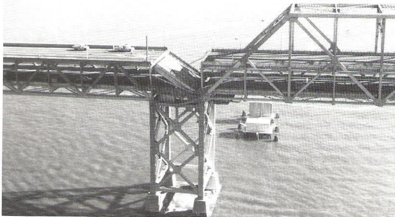
Pictures of the collapsed portion of the Bay Bridge were seen worldwide. (Photo by Ed Andersen, Caltrans)
